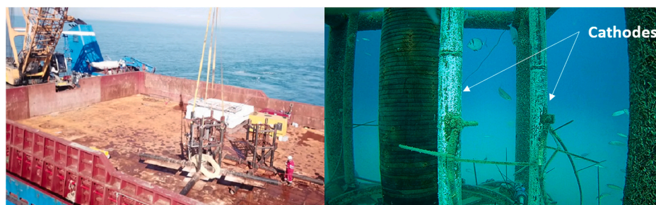
Fig. 4. Installation phase of the structure for the mineral deposition experiment (to the left) and view of the cathodes showing the mineral deposits on its surfaces after \frac{1}{2} month (to the right).
