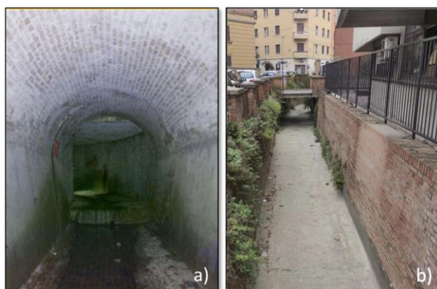
Figure 1. Two images of the course of Ravone torrent: a) a segment of the buried channel; b) an above ground portion.
