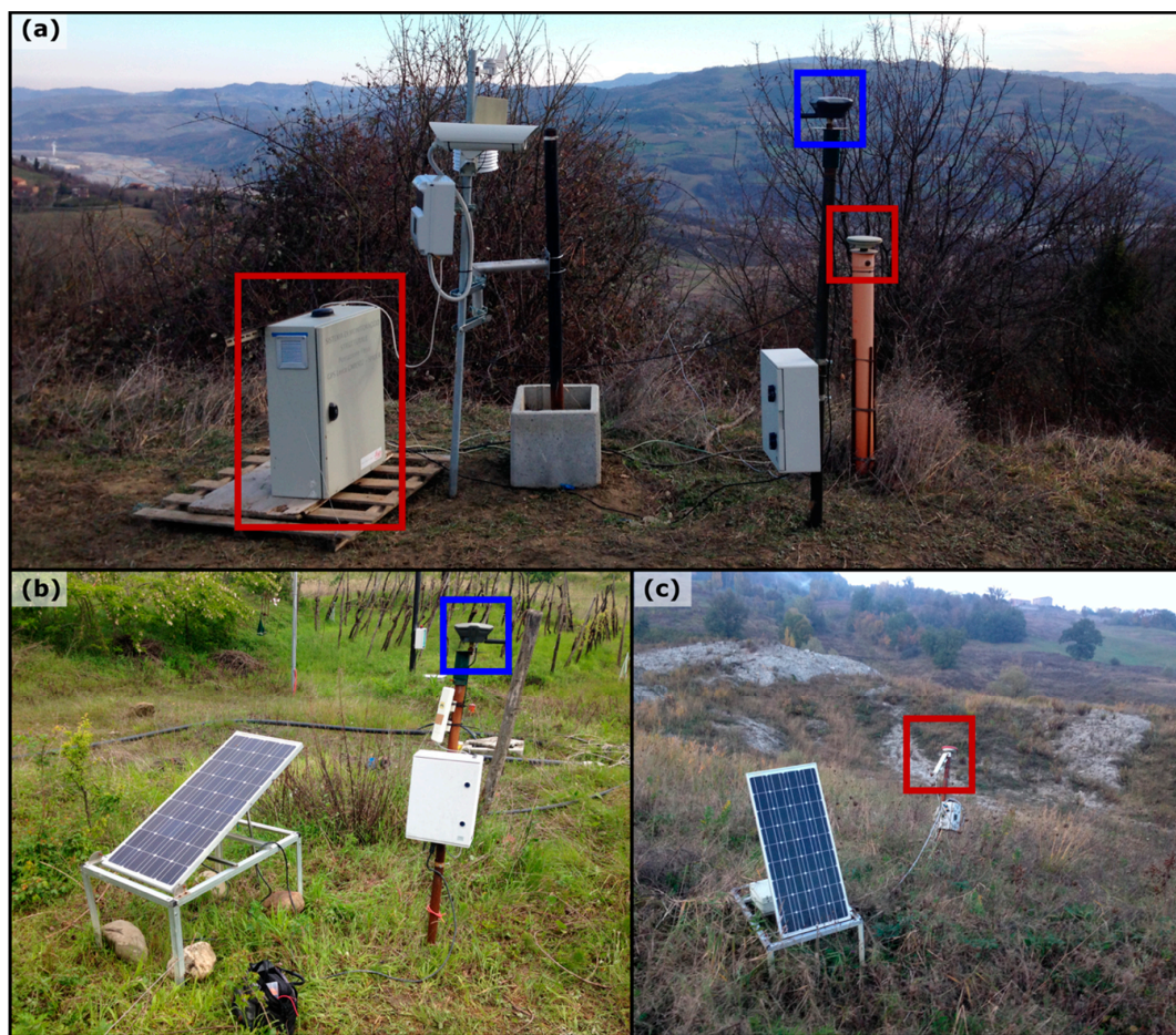
Figure 4. GNSS receivers installed at the Ca' Lita landslide. (a) Reference stations. Within the red squares are the Leica post-processing unit (left) and the Leica double frequency receiver on the right (model GMX902). In the blue square is the Emlid single frequency low cost receiver (model Reach RS) acting as a reference station. (b) Reach RS receiver is installed as ROV3b rover unit and its photovoltaic power unit. (c) Leica GMX901 receiver is installed as ROV2b rover unit and its photovoltaic power unit. During period "a", ROV1a, ROV2a and ROV3a were equipped with Leica GMX901 receivers. During period "b", ROV1b and ROV2b were equipped with Leica GMX901 receivers, while ROV3b was equipped with the low-cost Emlid Reach RS.
