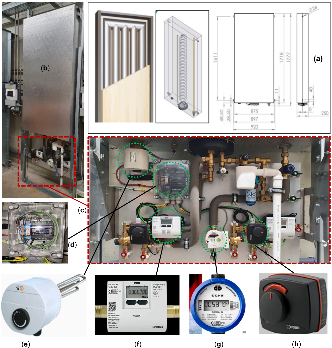
Fig. 3. Characteristics of the e -TANK system: Schematic and dimensions (a), storage prototype (b), hydronic unit (c), control cabinet (d), auxiliary electrical heater (relay) (e), ultrasonic heat meter (f), cold-water flow sensor (g), and three-way diverter valve + actuator (h).
