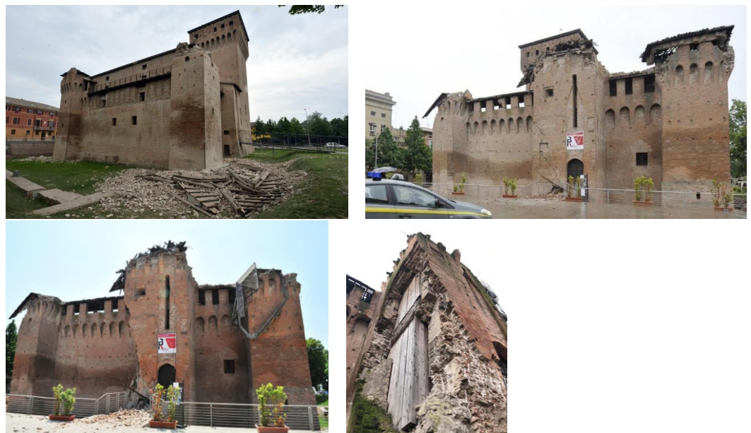
Figure 6. South-west corner after the first earthquake; the tower completely lost the last floor. The north front after the first earthquake: re-roofs and the corner of the north tower are still in place. The north front after the second shock, with the collapsed corner of the north tower. Credits: Repubblica Bologna. First aid intervention against the collapse of the whole tower after the expulsion of the corner. Credits: Comes Studio Associato.
