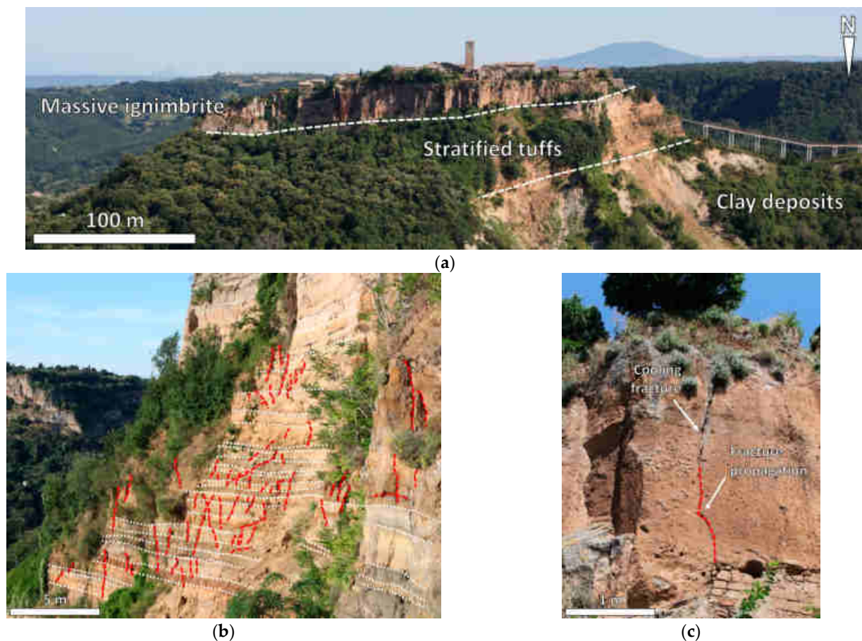
Figure 10. Rock mass and slope damage at Civita di Bagnoregio: (a) View of the volcanic plateau. Note the varying behavior of the materials that characterize the area, particularly the landslide developing in the clayey deposit. White, dashed lines mark the boundaries between the different materials. (b) Slope damage features (dashed red curves) affecting the stratified tuff, inducing a decrease in the overall rock mass quality that, in turn, affects the failure and deformation behavior of the slope. (c) Brittle damage, in the form of a fracture propagation from the tip of a cooling fracture, in the massive ignimbrite.
