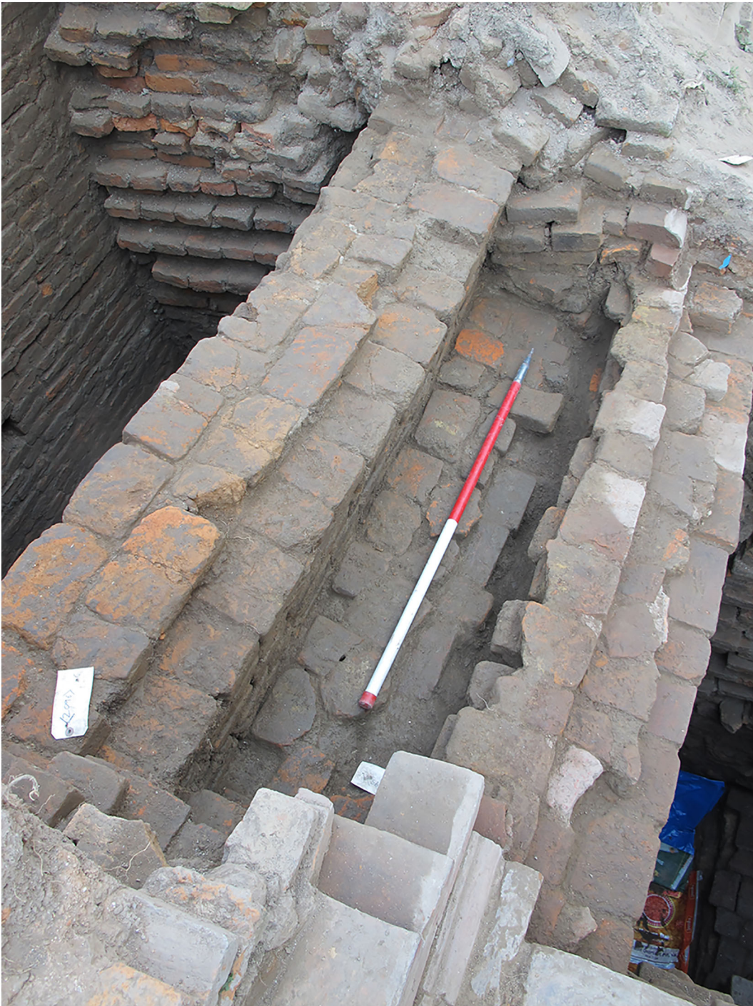
Fig. 7 Deformed and tilted wall, with later bracing, at Jaisidewal Temple (image: Keir Strickland)
