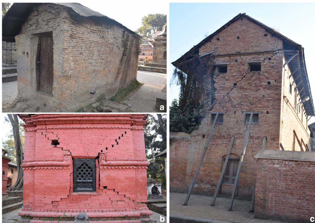
Fig. 3 Tilted wall at a structure at Mrigasthali in Pashupati (a); ‘X’ fracture through a brick built shrine at Mrigasthali in Pashupati (b); shear cracks through one of the walls within Bhaktapur Palace Complex (c)
