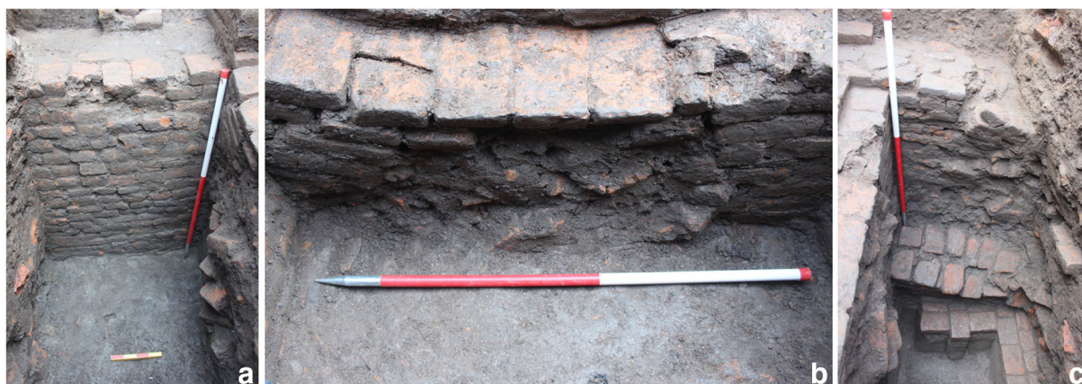
Fig. 8 Trench to the southwest of Jaisidewal Temple, with sequence of brick walls exhibiting shear crack and slight extrusion (a); tilting and collapse (b); crack and collapse of upper wall; and tilting of lower wall below (c)
