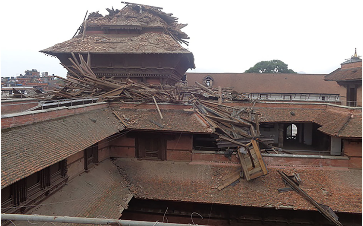
Fig. 2 Damage to the nine-storey palace in Hanuman Dhoka after the 2015 Gorkha Earthquake (image: Kai Weise)
