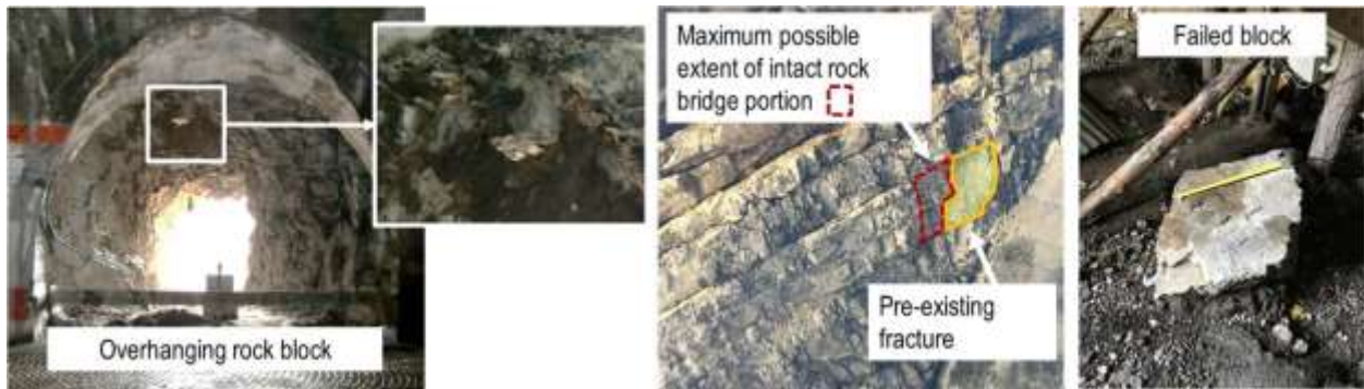
Fig. 4 Pre- and post-failure images of a rock block whose stability was apparently controlled by the presence of rock bridges
