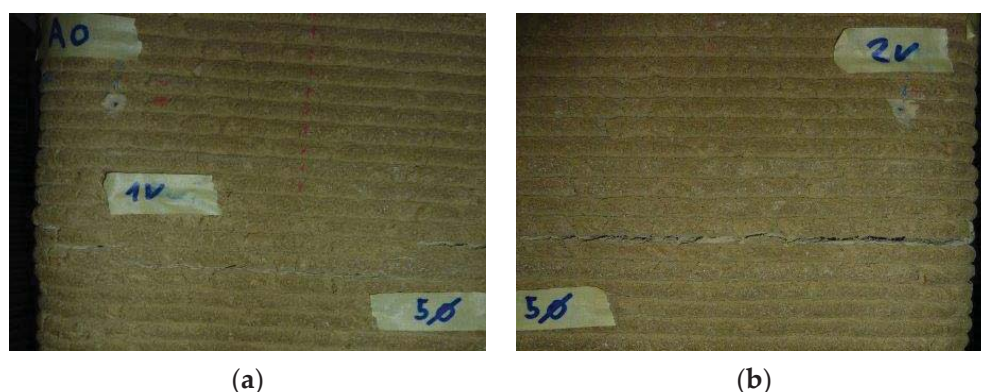
Figure 11. Details of the detachments between the horizontal layers of the side to the left of the operator: (a) left detachment, which reaches edge 1; (b) right detachment, which reaches edge 2.
