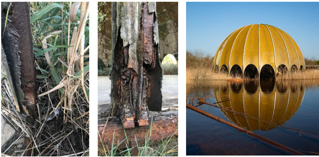
Fig. 11 a) Deterioration of the fibreglass layer that initially wrapped metallic tubes; b) corrosion of metallic framework near the base (two joined flanked tubes and their connection to the basement can be seen); c) rising of the level of ground water during the rainiest periods (courtesy of Antonello Zoffoli).
