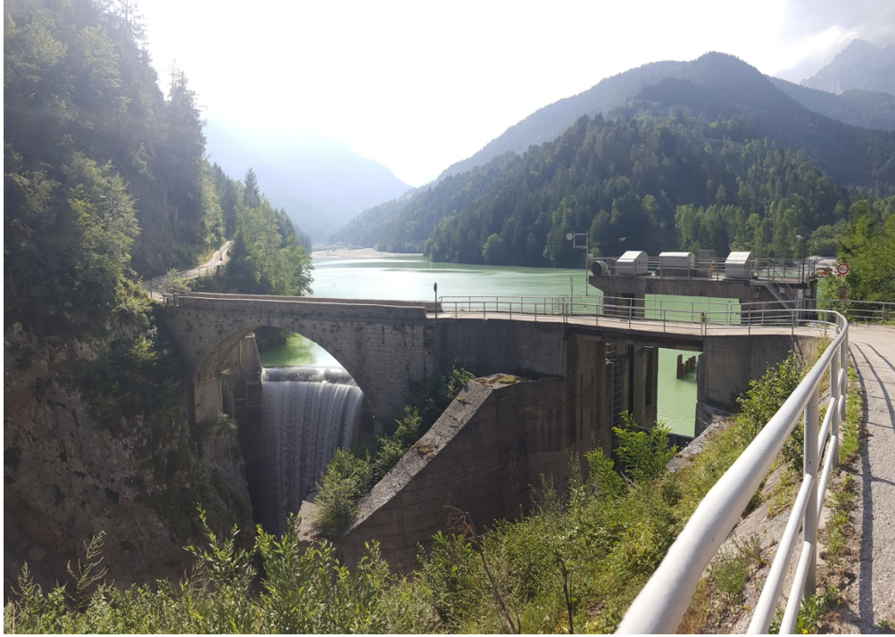
Figure 3. The dam and the intake structure of Valle di Cadore (photo taken by the authors on 11.08.2019).
