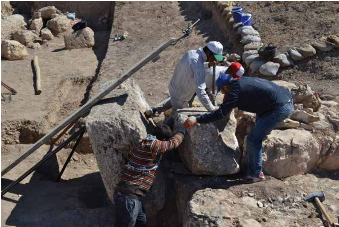
1. Late Bronze Age I southern tower (phase 10): the eastern orthostat during the restoration process.
