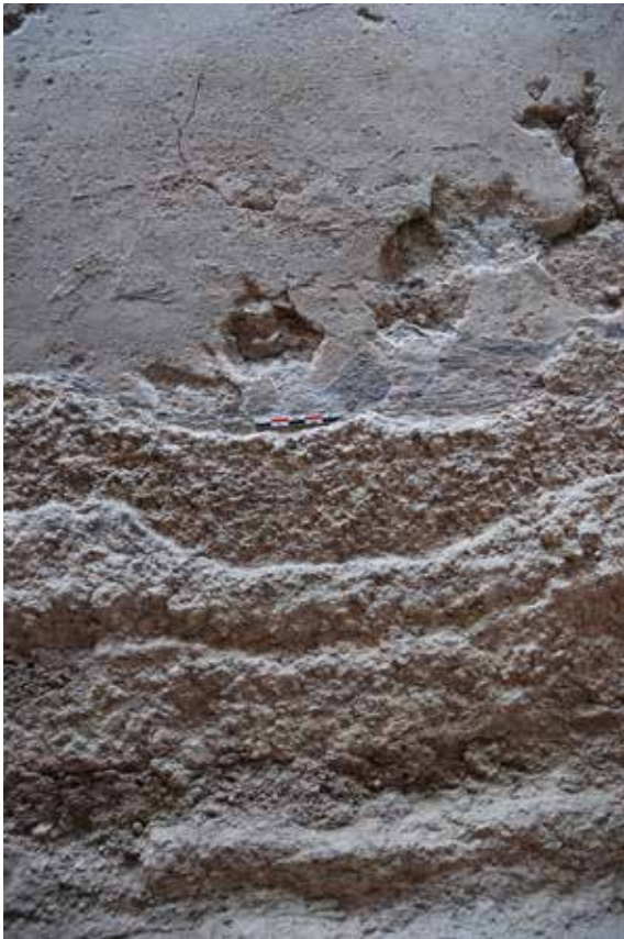
1 Detail of the inner waterproofing of the Roman water conduit D.2600c (phase 3).
