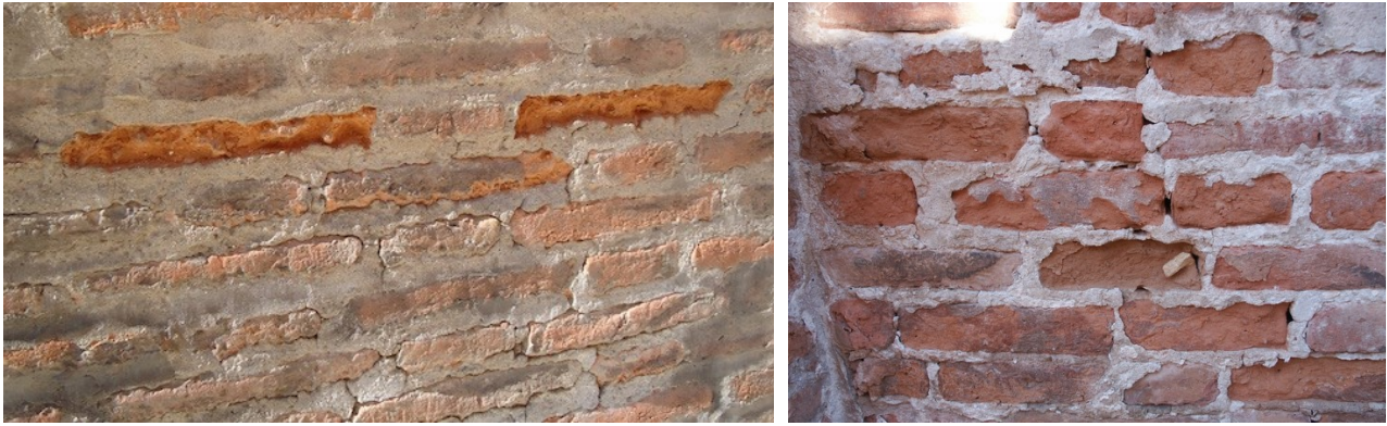
Figure 15. Increase of bricks deterioration in correspondence of scarcely permeable repointing mortars, boosting the water transport through the bricks (on the left: complex of the Corpus Domini church, Bologna, Italy; on the right: S. Maria delle Consolazioni church, Este, Italy).
