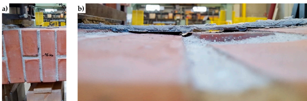
Figure 44. Delamination of the compressed CFRP strip: (a) length of the crack for the delamination load on the compressed side (15 kN) and (b) detail of delamination, just above the crack.
