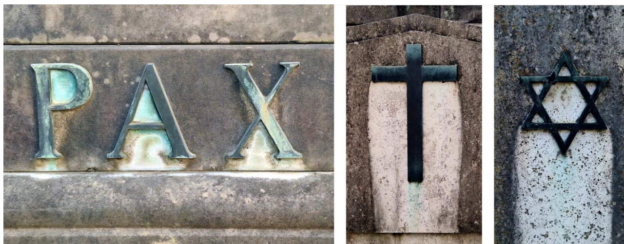
Figure 1: Examples of biodeterioration (the dark areas are affected by biological growth, while in the pale areas the biological growth is inhibited by leaching of copper ions from letters and symbols).
