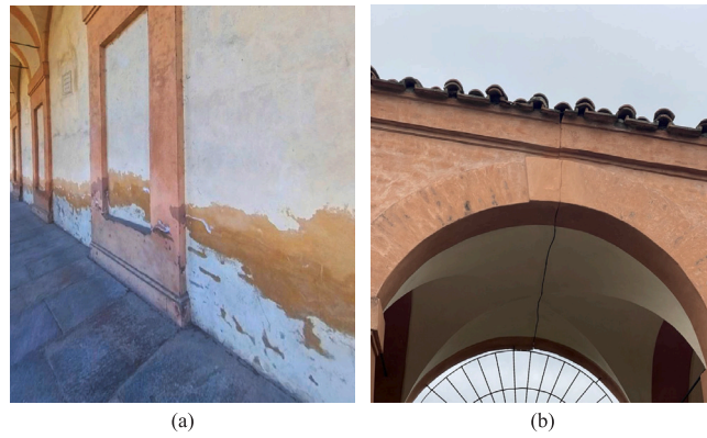
Fig. 17. Pictures of structural details: (a) efflorescence caused by rising damp between Mysteries IV and V, documented in 2020, (b) structural disconnection between Mysteries IX and X, documented in 2025.
