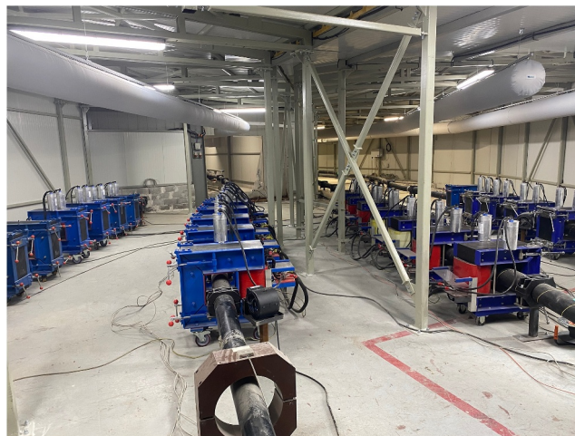
FIGURE 1 | Heating transformers in the PQT loop of a 525-kV DC-XLPE cable system. Two loops are under test, one with a land cable (left), the other with a submarine cable (right) (Courtesy Hellenic Cables, Greece).
