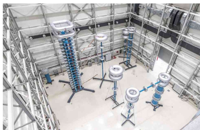
FIGURE 6 | Combined DC and impulse voltage test system (Courtesy HIGHVOLT Prüftechnik Dresden GmbH, Germany).
