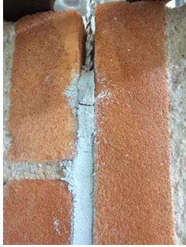
Failure mode B*: bar pull-out with local fracture of the mortar
