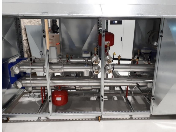
Figure 3. Inside of the prosumer substation.
