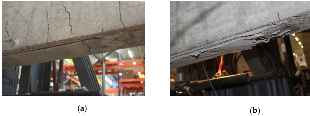
Figure 11. Photos of the anchors at the end of the test for specimens (a) FB_2400_150_MD_1L_B250 and (b) FB_2400_150_MD_1L_ER250.
