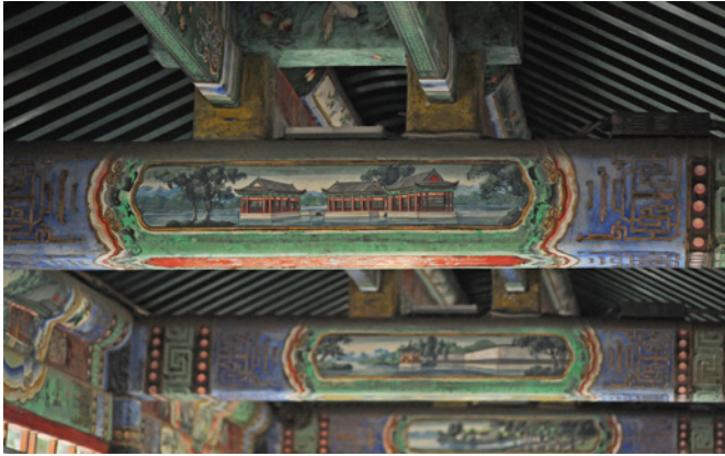
Fig. 1. Detail of the wooden roof structure of the Long Corridor of the Summer Palace or Yiheyuan in Beijing © 2011, C. Mazzoli.
