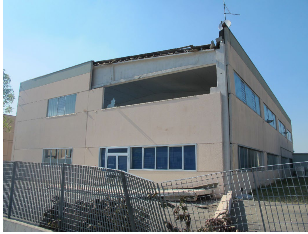
Fig. 2. Typical damage observed in precast buildings struck by the Emilia earthquakes: (a) plastic hinge at the base of a column; (b) loss-of-support of a simply-supported roof slab from main girders; and (c) out-of-plane overturning of RC cladding panels.
