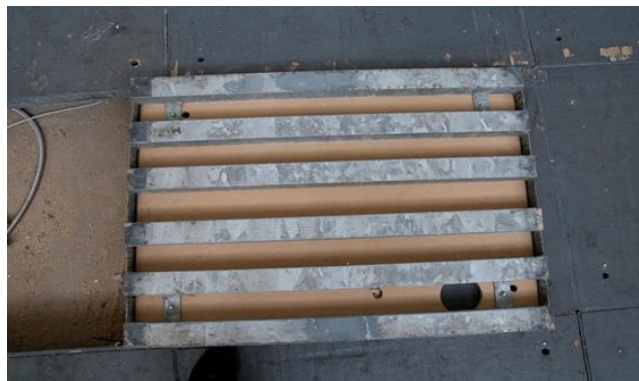
825 826 Figure 8. Detail of the reinforcing metal mesh in the floor of the hall.
