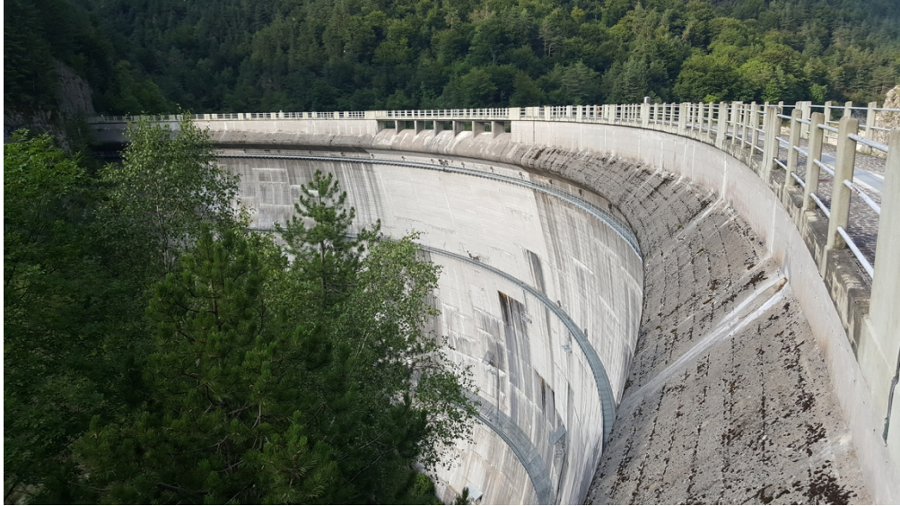
Figure 1. The spillway of Val Gallina Dam (photo taken by the authors on 11.08.2019).
