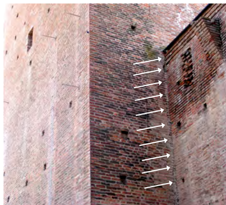
(b) Mastio - East wall joint: poor tothing quality
