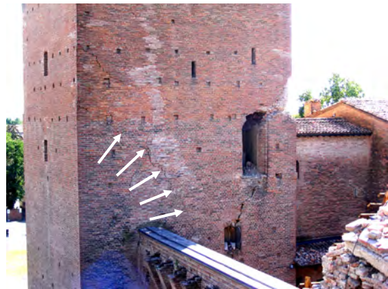
(b) Crack pattern
