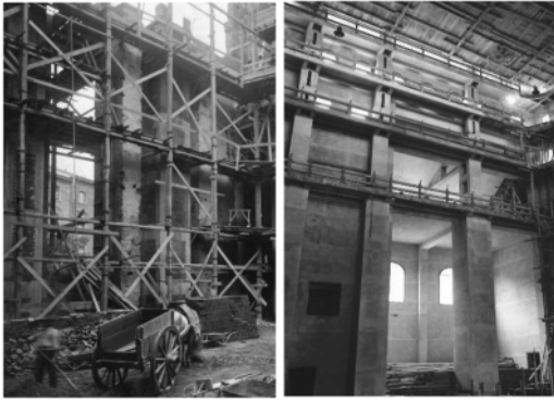
Figure 13, 14. The reinforced masonry pillars. –The pillars with the Vierendeel shape. Donati & Zanichelli Company's private archive.
