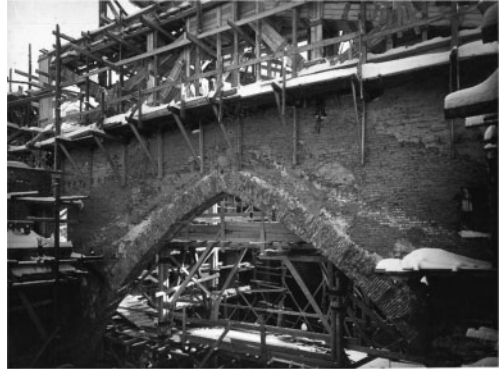
Figure 15. The consolidation and caging works of the wall. Donati & Zanichelli Company's private archive.
