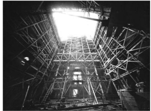
Figure 10. The lifting towers of the metal beam. Donati & Zanichelli Company's private archive.
