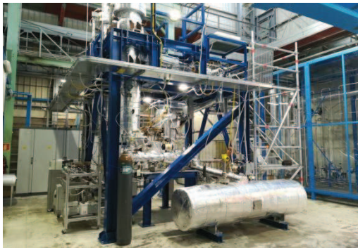
Figure 2: TRIEX-II facility installed at C.R. Brasimone.
