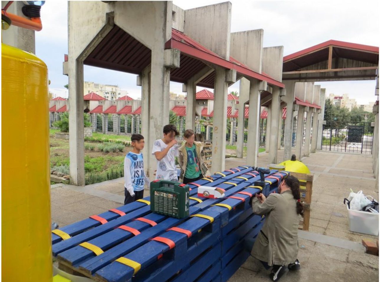
Figure 12: Orto Urbano, Ponticelli: Construction of a water harvesting and filtering facility in a community space with participation of the local community.
