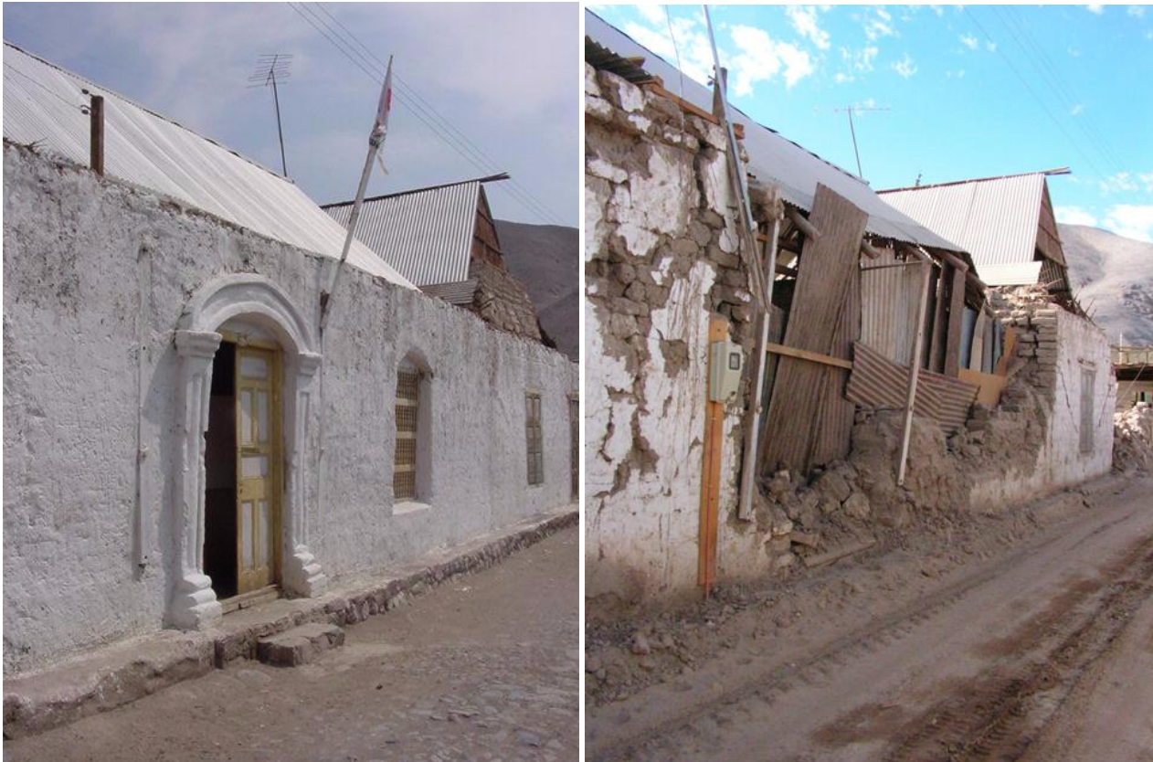
Figure 2: Before and after the 2005 earthquake in San Lorenzo de Tarapacá. Source: www.proyectotarapaca.org
