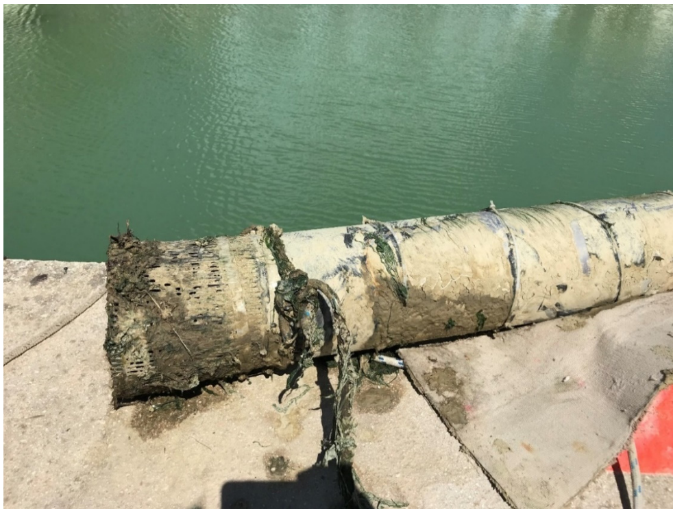
Figure 9. Fouling of the external filter of the pump; picture taken on 2 of May 2019, before cleaning.
