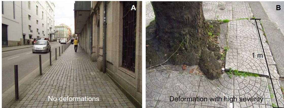
Figure 27: [A] Pavement with no deformations (Rua Magalhães Lemos, Porto) and [B] pavement with deformations due to tree roots (Rua Campo Alegre, Porto). Photos by Fernando Fonseca, CTAC.
