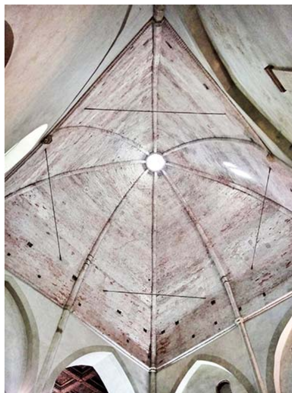
Fig. 11: Internal view of the dome of the baptistery of Saints Giovanni and Reparata in Lucca (Tuscany). Photo: F. Fantini
