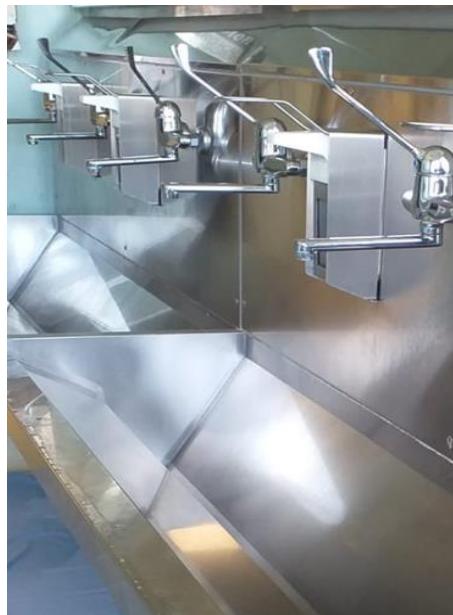
Figure 4. SHWOs with elbow-operated manual faucets without TMVs.
