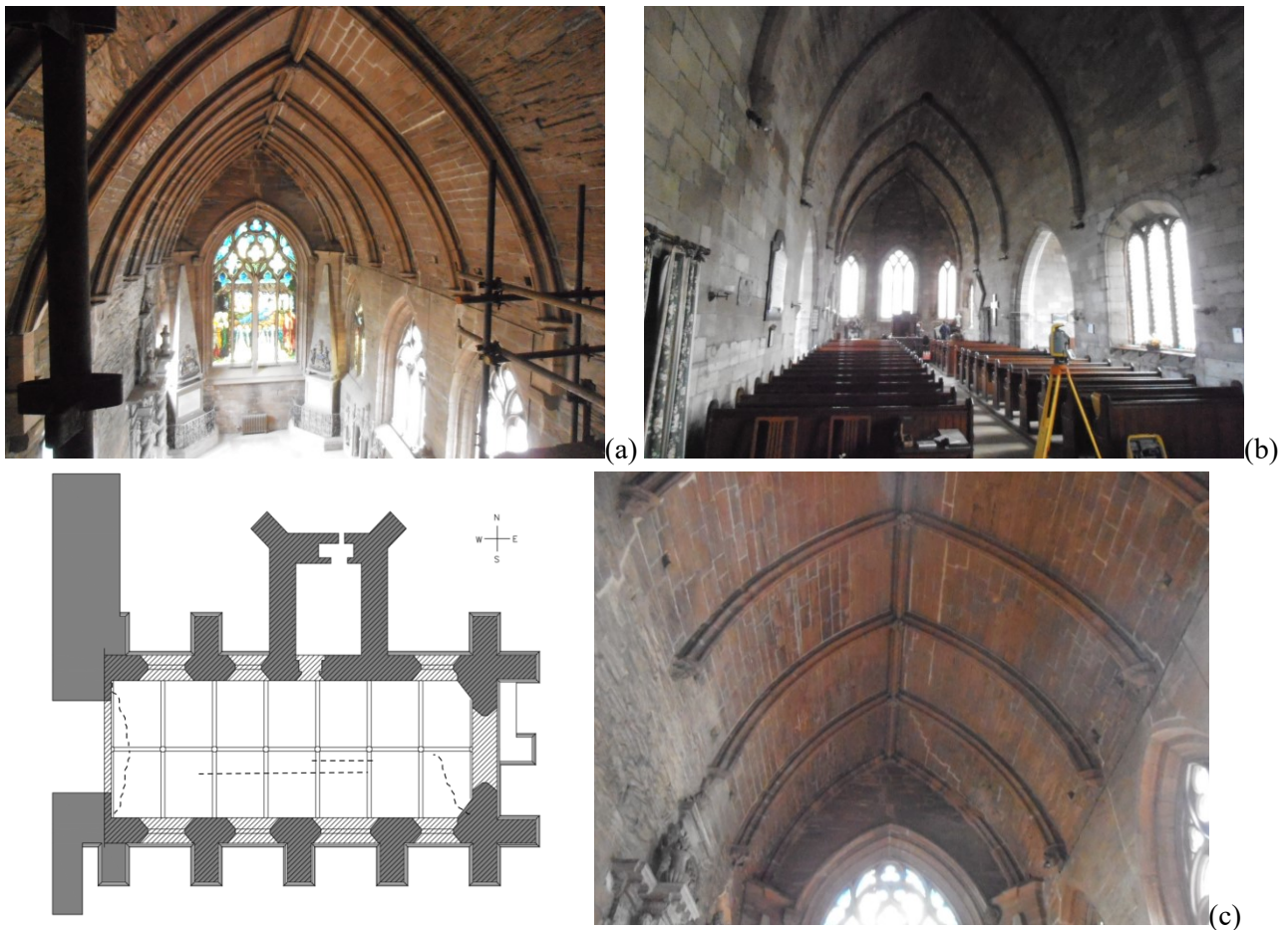
Fig. 1 – The earliest (a) (Bothwell 1398) and latest (b) (Ladykirk 1500) examples of barrel vaults in late-medieval Scotland churches. Crack pattern in Bothwell (c) due to deformation in the South wall from [27] and its appearance at the East end of the interior (following repairs in 2016), (settlement caused at the right-hand corner).
