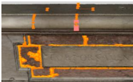
Figure 13. An example of the mapping of damaged areas, by means of direct identification and sketch on the 3D model of the basement.
