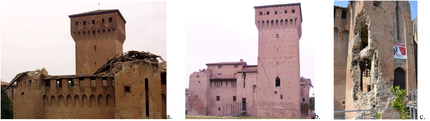
Fig. 4 - Collapse of a minor tower's roof (a), damage pattern in the Mastio (b) and collapse in the north tower (c).
