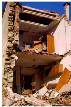
Figure 1. Collapse of a double-layered masonry wall [1].
