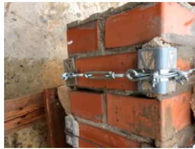
Figure 14. The fastening system along the lateral face of the brick wall (23 cm).
