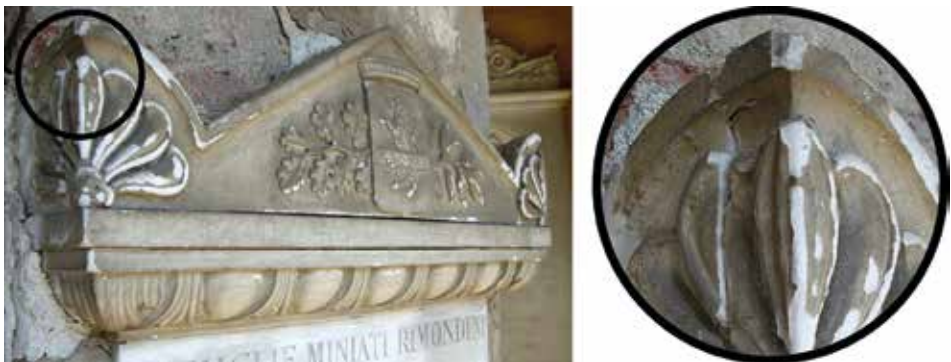
Figure 1: Example of marble decoration affected by sulfation (Monumental Cemetery in Bologna, Italy, XIX century). Beneath the gypsum surface layer (also incorporating some particulate matter), marble exhibits grain disaggregation
