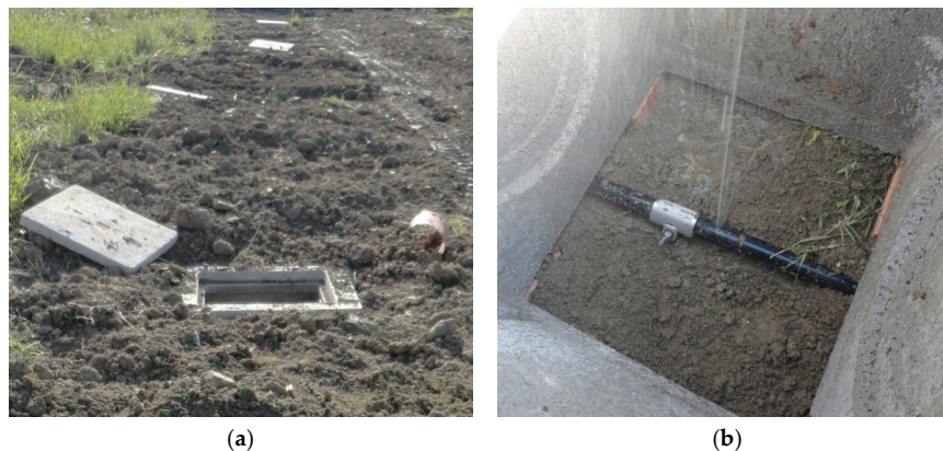
Figure 8. New setup: (a) buried pipeline with manholes installed; (b) active leak accessed through a manhole (plastic sack with soil temporarily removed to observe the leaking flow).
