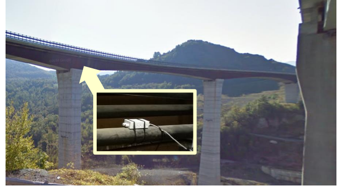
Fig. 8. Viaduct along an Italian motorway, where sensors deployed for structural health monitoring are attached to the internal tendons.
