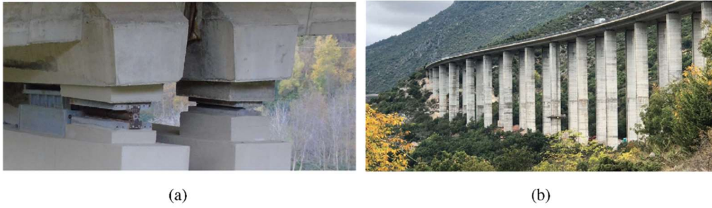
Fig. 4 – Detail of the supports (a) and side view of an A24 viaduct (b) [9]
