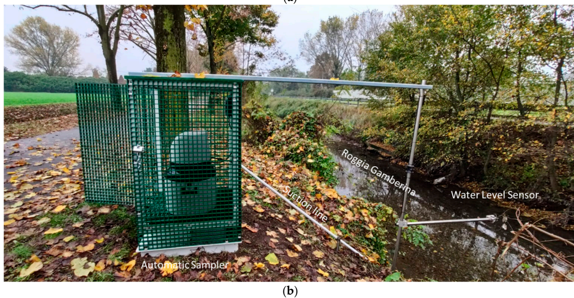
Figure 2. (a) Automatic sampler installation within the outlet of Basin 1. (b) Automatic sampler and water level installation within the Roggia Gamberina in Basin 2.
