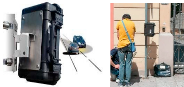
Fig. 3. (a) radar equipment used for speed monitoring (b) installation of the equipment to vertical signs
