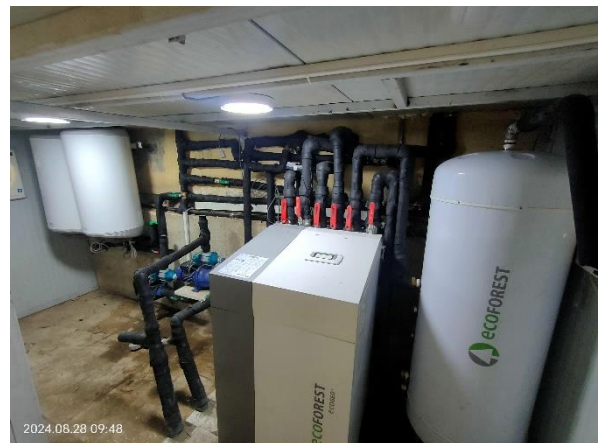
Figure 7: GSHP system installed at Cairo University.
