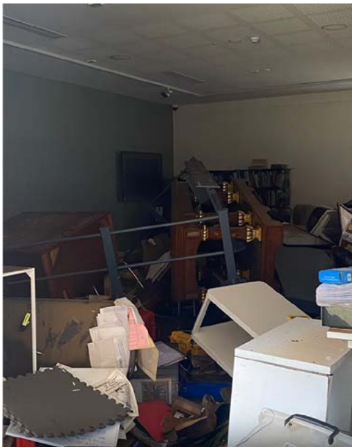
Figure 8. Damages to a room of the Art Gallery due to the flood and the fire.
