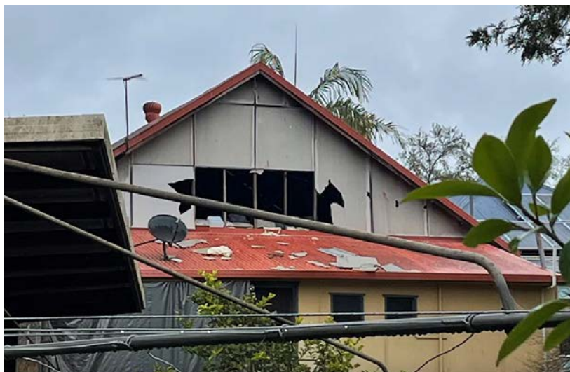
Figure 6. Damages to a third-floor roof attic in Lismore.
