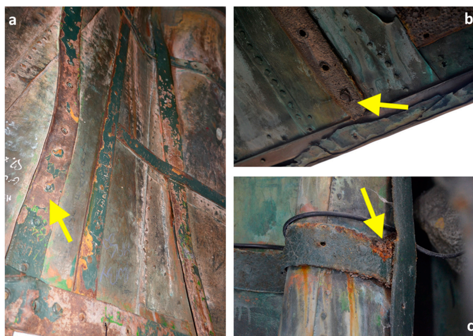
Figure 2. Examples of degradation patterns on iron elements. (a) Iron bars in good conservation conditions despite the degradation of the protective coating; (b,c) small areas characterised by severe corrosion surrounded by almost intact zones.
