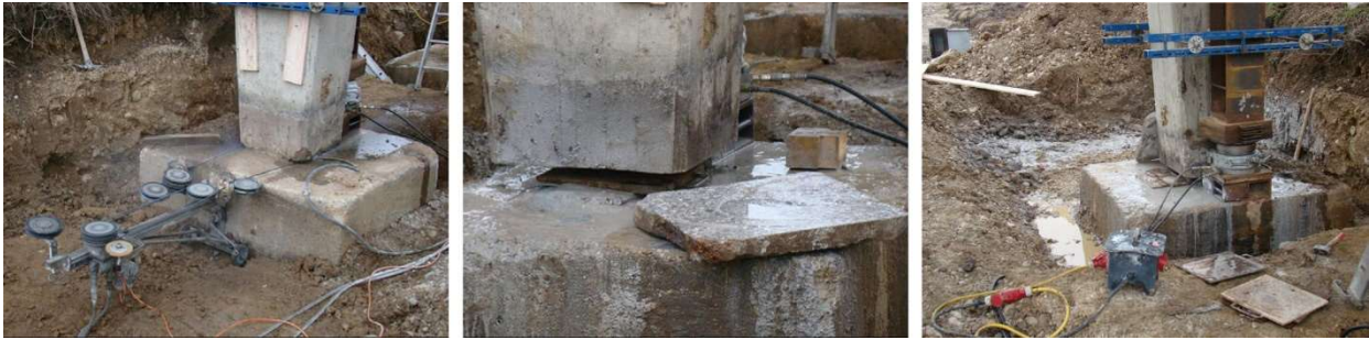
Fig. 7: Photographic documentation of the pier settlement process [72].
