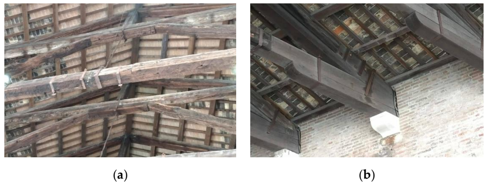
Figure 3. Construction details of the roof: (a) suspension of the tie element; (b) support on the masonry by a stone cantilever and barbican.
