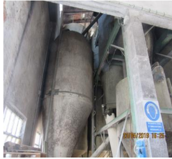
Fig. 5. Flour storage silo in a pork breeding farm.
