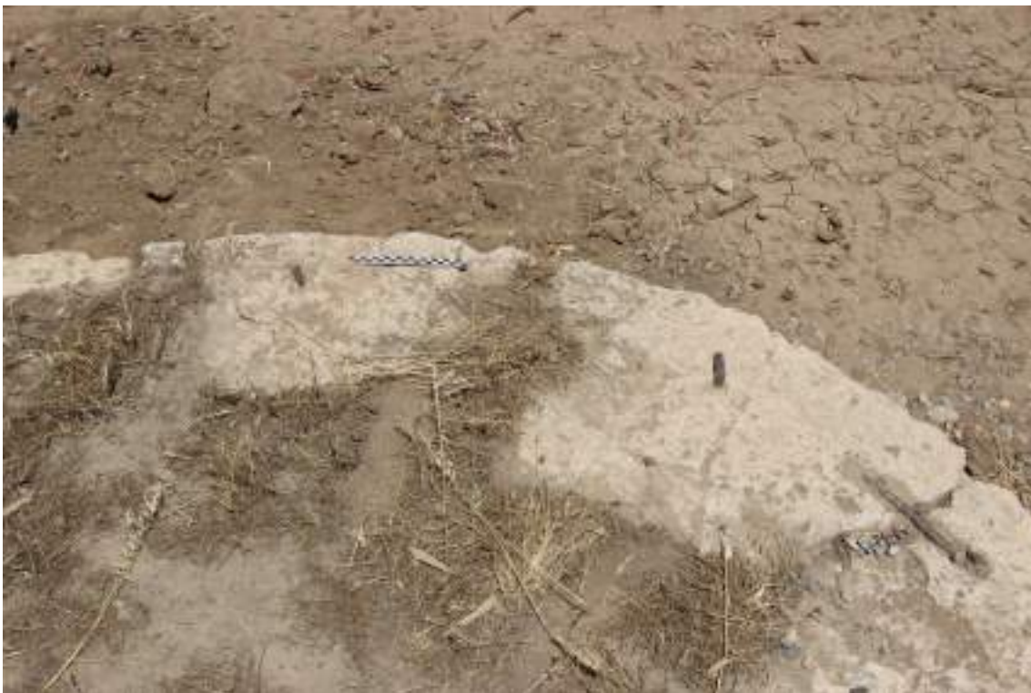
2. Iron plug protruding from a hole in a sixth course ashlar of Pier 3.
