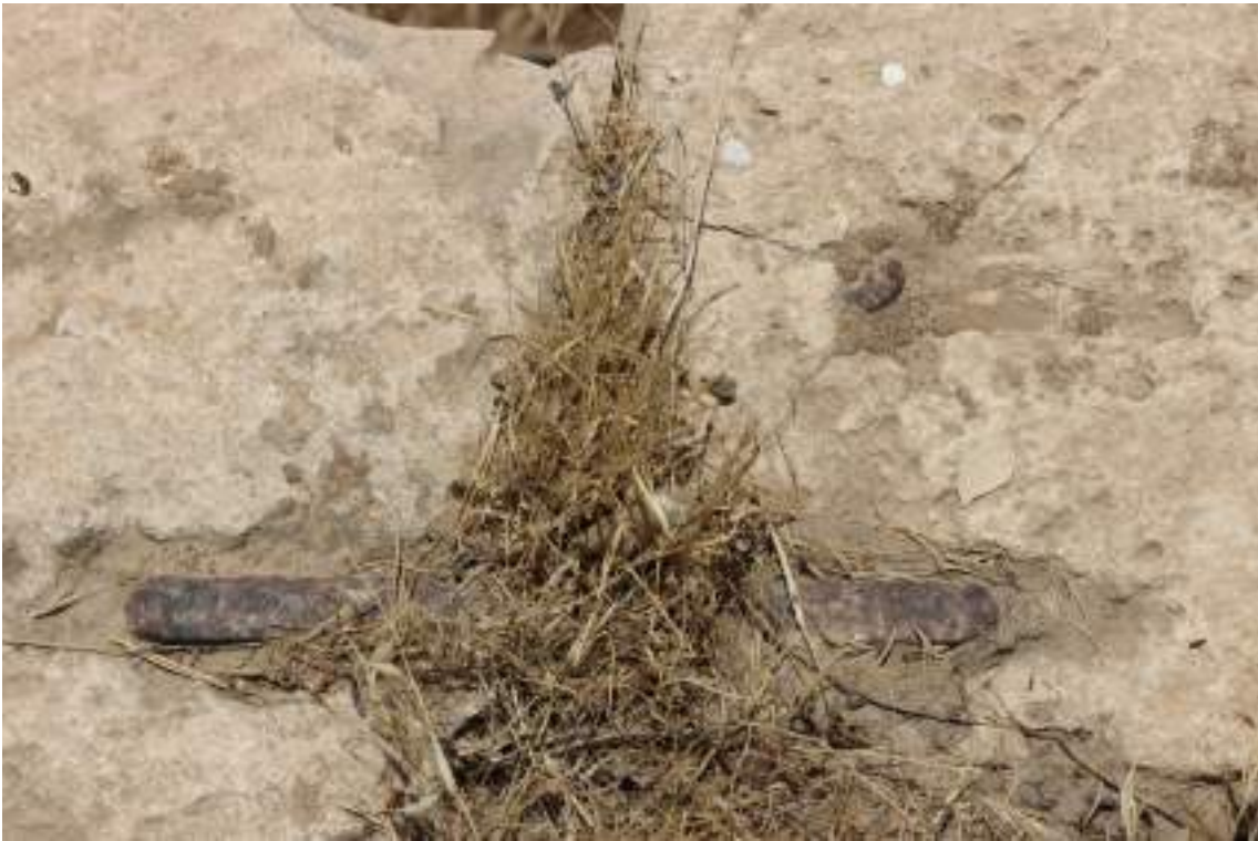
1. Close-up of a iron plug and a iron clamp.
