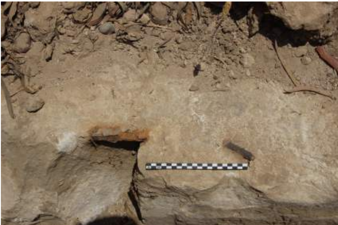
2. Pier 4: close-up of an iron clamp and peg.
