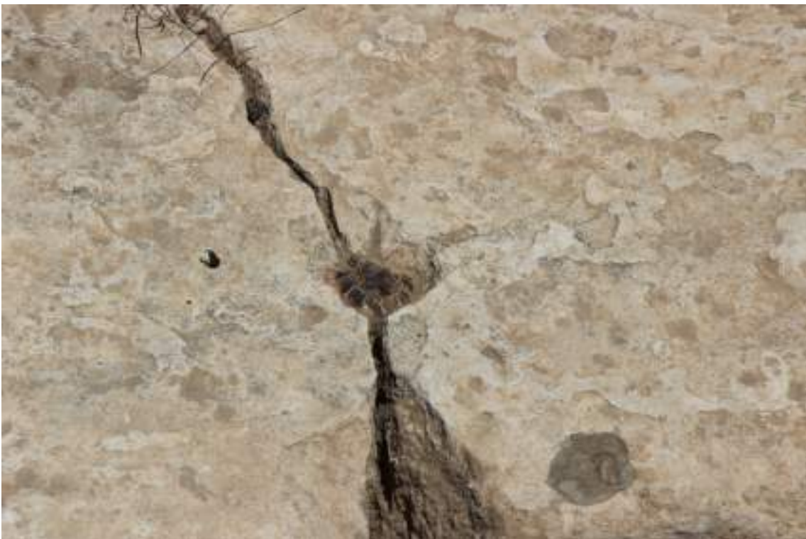
2. Iron rod visible inside the hole.
